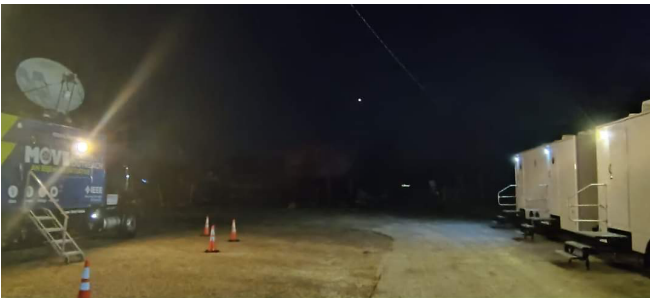
MOVE-2 providing lighting for showers and restroom facilities for residents
